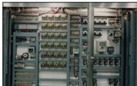
Pre-wired Electrical Control Panel
