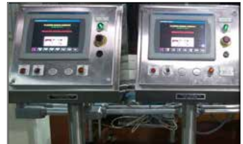
VFD Variable Speed Controls and Allen Bradley PLC
