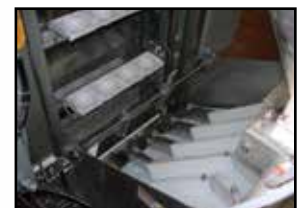
Pneumatic Flapper Gate Transfer
