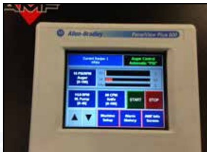
Operator Interface Panel
