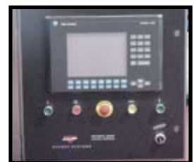
Operator Interface Panel
