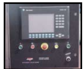
Operator Interface Panel
