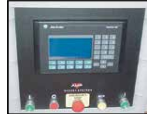
Operator Interface Panel
