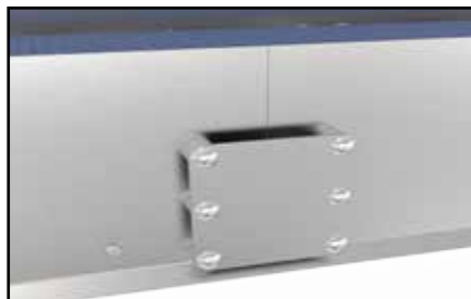
Junction Plate Stands Off
