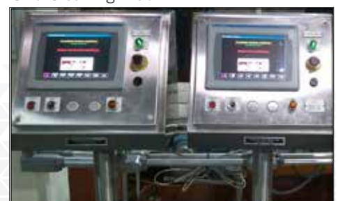
Operator Control Station
