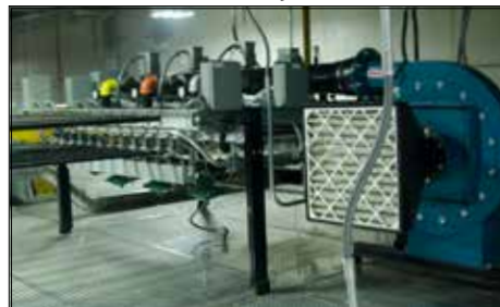
VFD Controlled Fans
