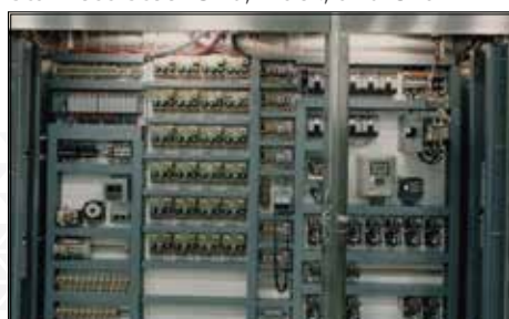
Pre-wired Electrical Control Panel
