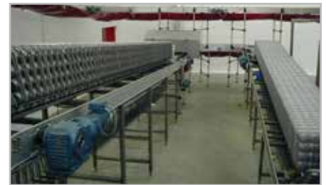
Two Separate Conveyor Sections
