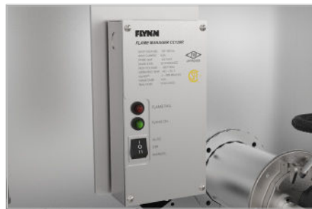
DSI and Burners Distributed I/O Panel
