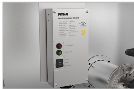
DSI Distributed I/O Panel and Burners
